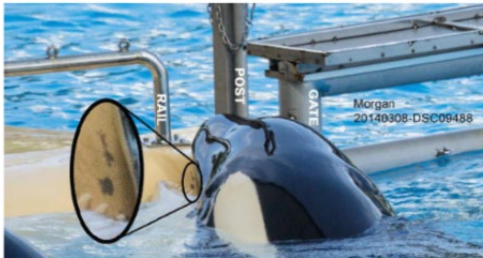
Figure 25b. Morgan chewing on the concrete in the east tank. Despite the water level being higher in this 2014 photograph, a small section of concrete can be seen as damaged (see enlarged area). Note the gate, post and safety rail positions labelled in both photographs to allow cross referencing of Morgan's position and the area damaged in Figure 25a. The wooden maintenance separators are not present in this 2014 photograph, rather the water from the west tank is visible.
